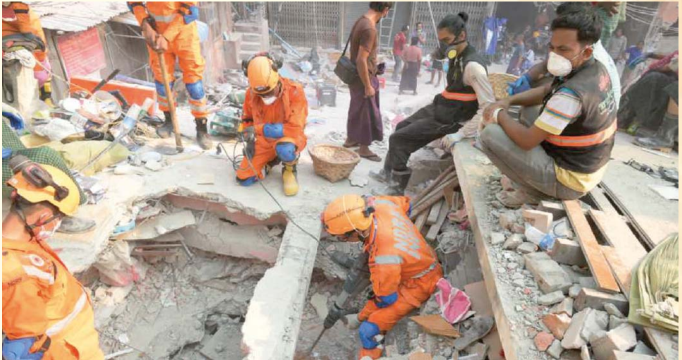
NDRF Rescuers conducting Search and Rescue (SAR) Ops amidst collapsed structures in Mandalay Region in Myanmar – April 2025.
